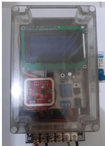
Figure 4. Individual electric consumption meter
